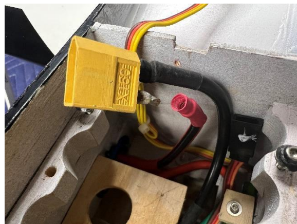
Broken Wire at the Battery Connection
