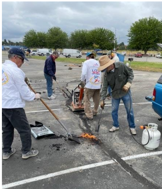
Valley Circle Burners President Dave Hull (Straw hat) trying not to burn down the circle. Seriously, Dave and his crew are patching the massive cracks as seen in the top left picture.
